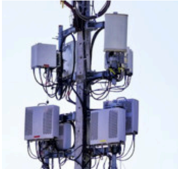
Above: 5G antenna tower
